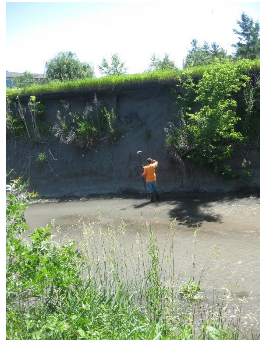
Example of unsafe tall banks affected by accelerated bank erosion that continues to create unstable conditions and drop trees. The project plans to shape milder slopes to make riparian areas safer and more stable.
